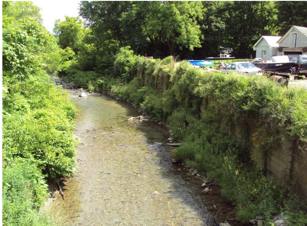
Photo 30 The Little Hoosick in the hamlet of Berlin. The crib walls were built after massive flooding in the 1950s.
