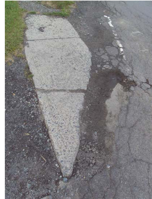
Photo 6 A portion of the sidewalk along Park Avenue that has been partially covered by asphalt and gravel.
