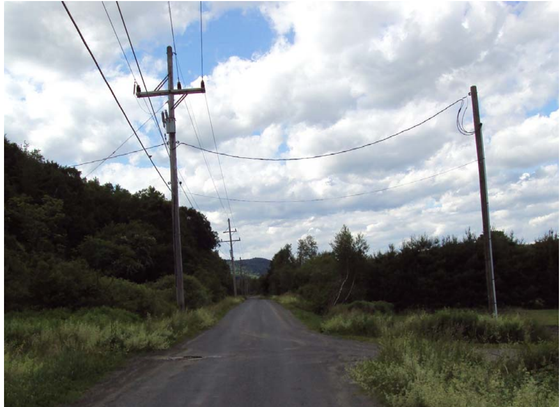
Photo 14 The 15 kV power line feeding the businesses of Berlin
