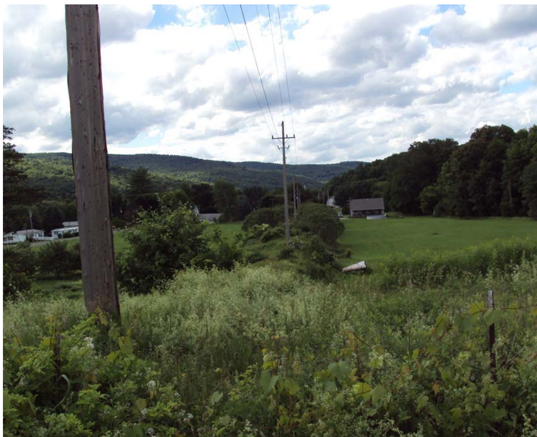
Photo 5 The 15 kV feeder line to the hamlet of Berlin running along the old rail bed.
